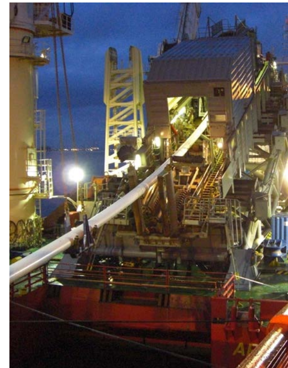
Onsite post-heating for the oil and gas industry is a growing application area for ENRX.
