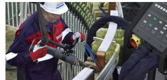
An ENRX Minac brazes generator windings. Minac's mobility and the handheld transformer let operators access hard-to-reach areas.
